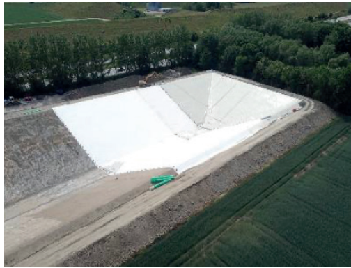
Figure 56: Diffusor connection (left); Laying the liner in Høje Taastrup (Source: Gquadrat) (right)
