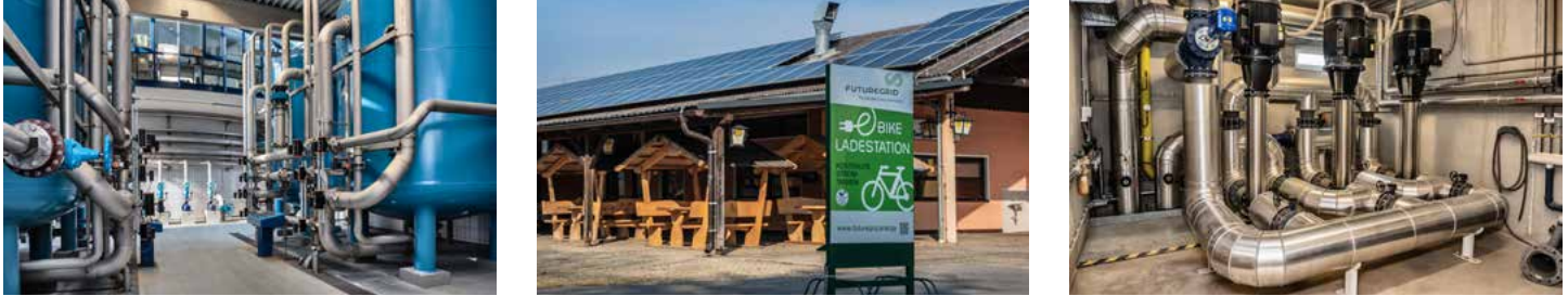
From L to R: critical infrastructure (water supply), photovoltaic e-bike charging station, power-to-heat equipment at biomass heating plant, photos: act4.energy
